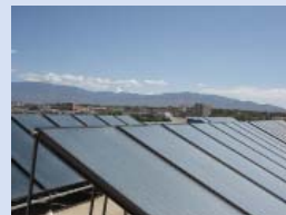
The solar panels are set back and installed at a low angle to the roof top so as not to be seen from the street.
