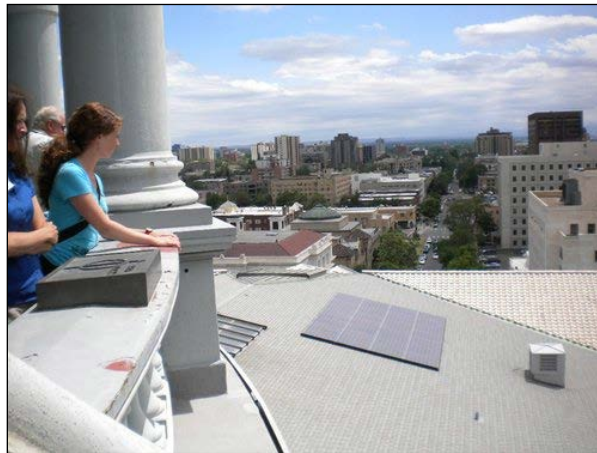
Figure 7. PV Panels on Denver Capitol Photo by Eliza Hotchkiss, NREL/PIX 18594
